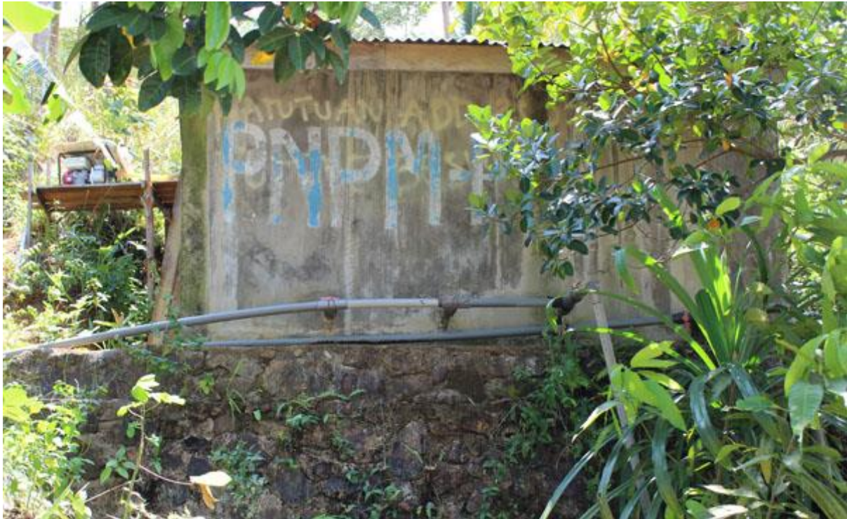
Figure II-15. One of the PNPM project at Air Sena, fresh water supply system
