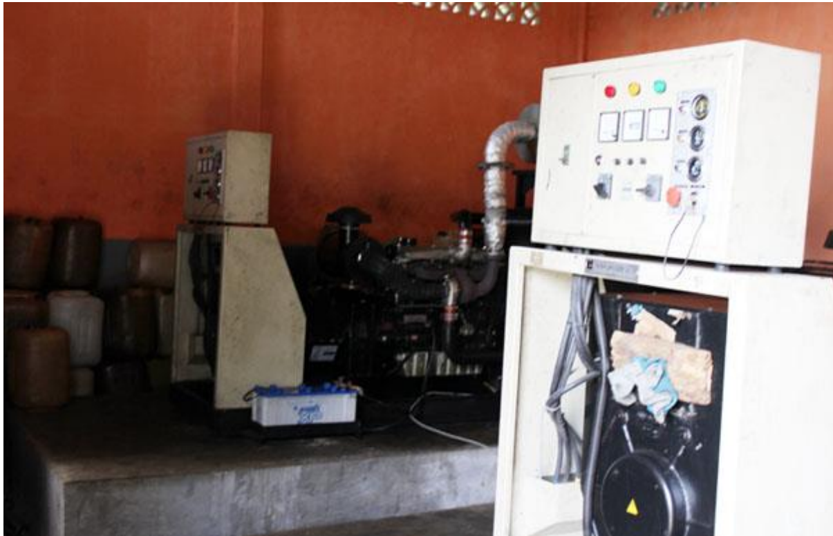
Figure III-2. Diesel Power Plant at Air Sena Village
