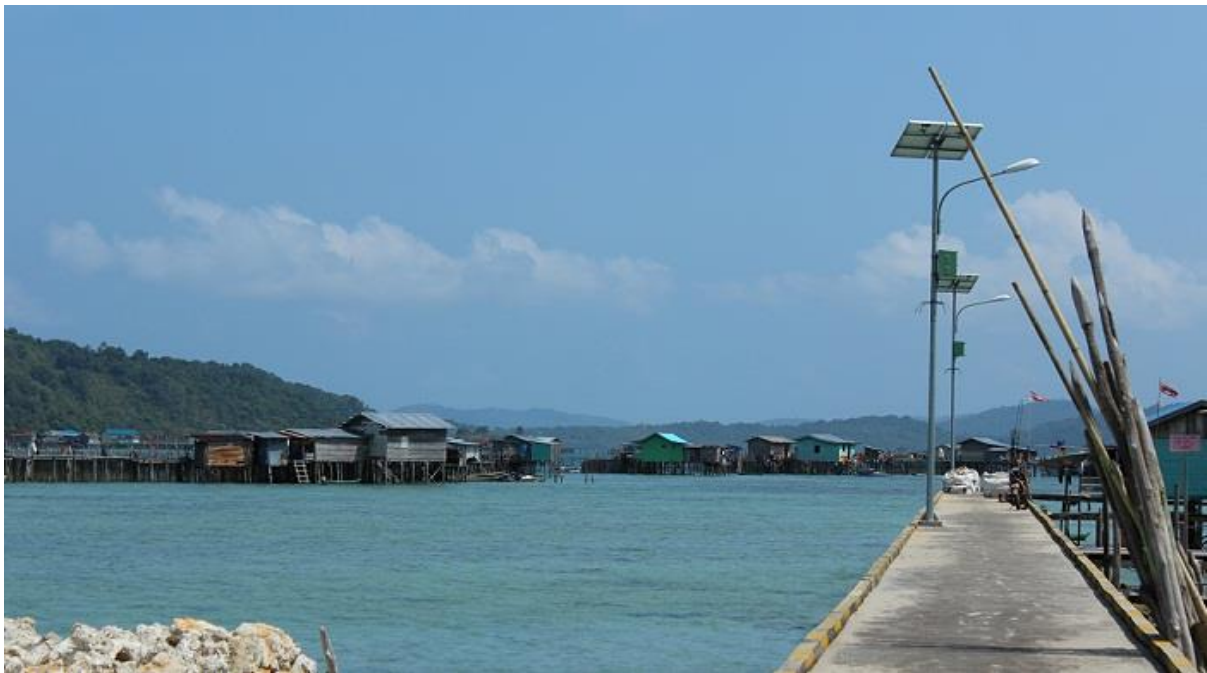
Figure III-5. Solar photovoltaic street lighting system at Air Sena
