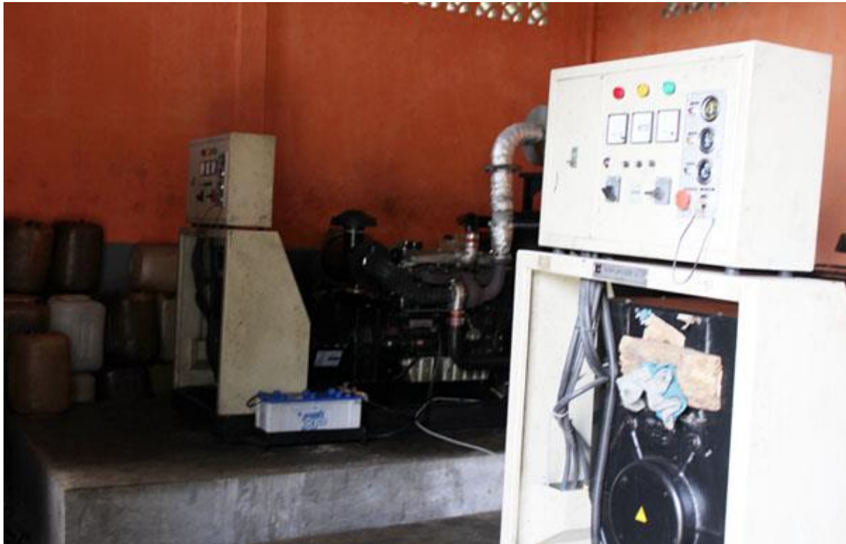
Figure III-2. Diesel Power Plant at Air Sena Village
