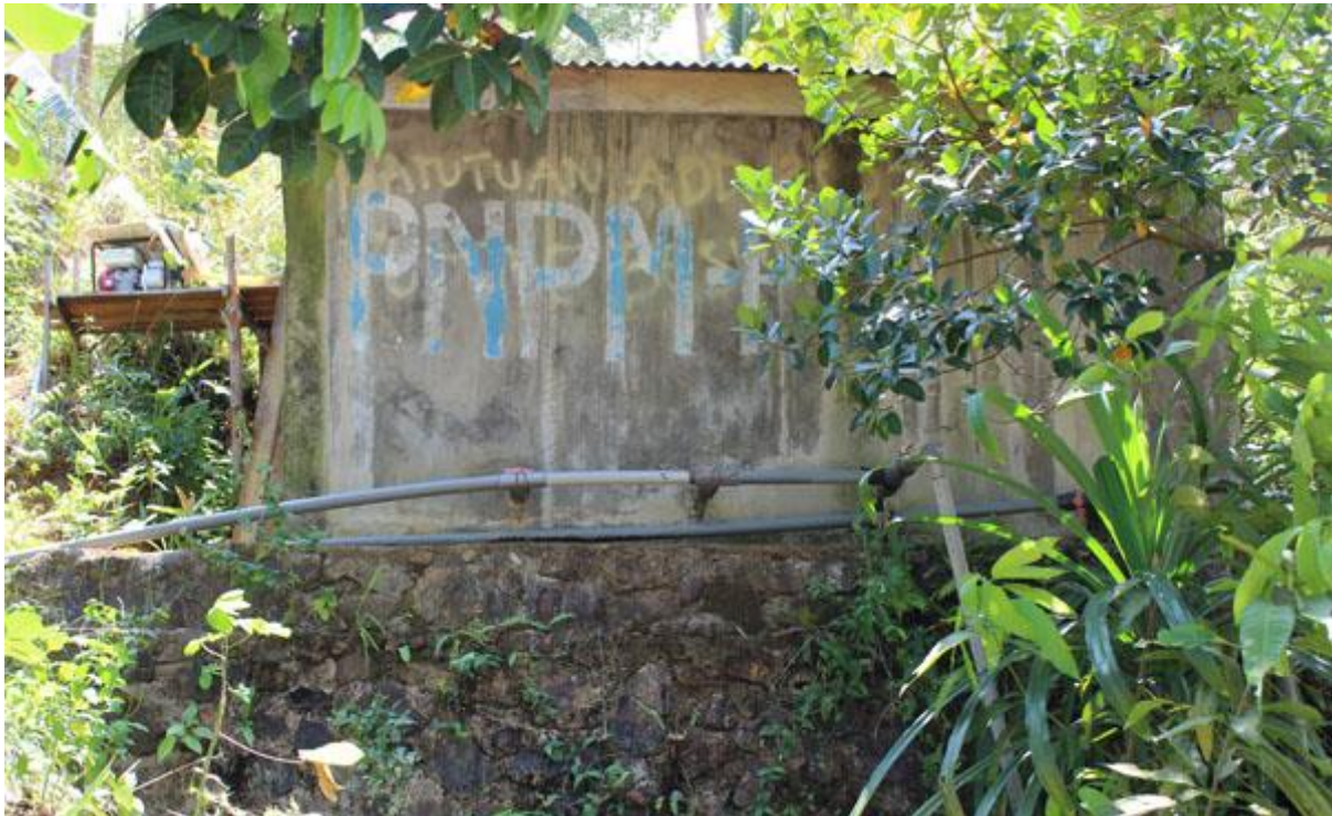
Figure II-15. One of the PNPM project at Air Sena, fresh water supply system
